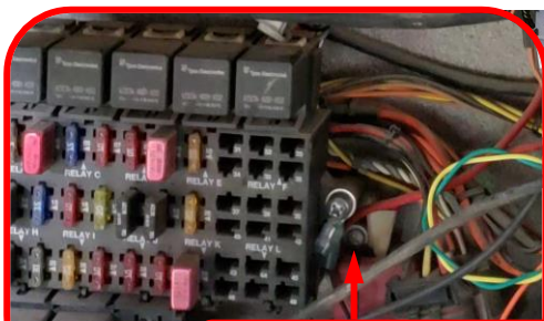
Constant Battery, Ignition, and Ground Connections
