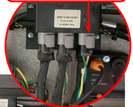
Figure A: 6-way Chassis CAN Connector —If 6-way bus not plugged in here, see Figure B for 3-way Gray Splitter.
