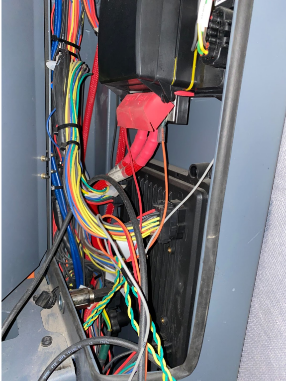
Behind the driver's seat for constant battery, ignition, and ground connections.
